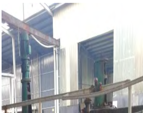
中间渣暂存库 (625m 2 )
